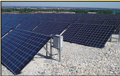
The 500-kilowatt array in Camden County, N.J., is providing 105% of expected output.
